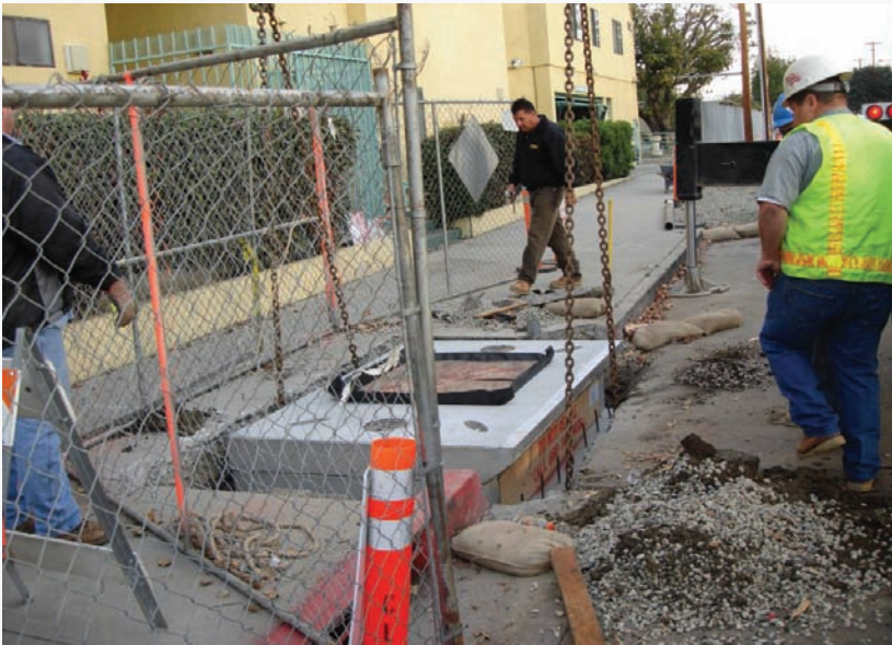
Figure 3. Bacteria™ Advanced Bioretention Technology Installation for Urban Streetscape Retrofit Project in Marina Del Rey, CA.
