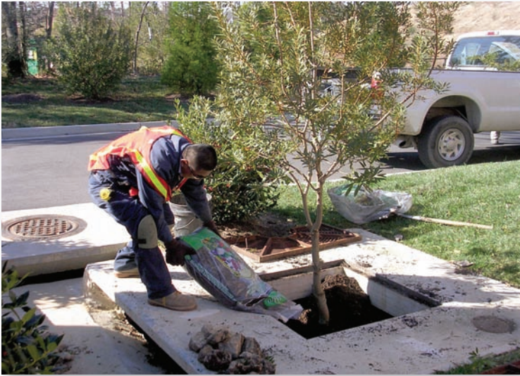
Figure 4. Filterra® Stormwater Bioretention Filtration System Maintenance.
